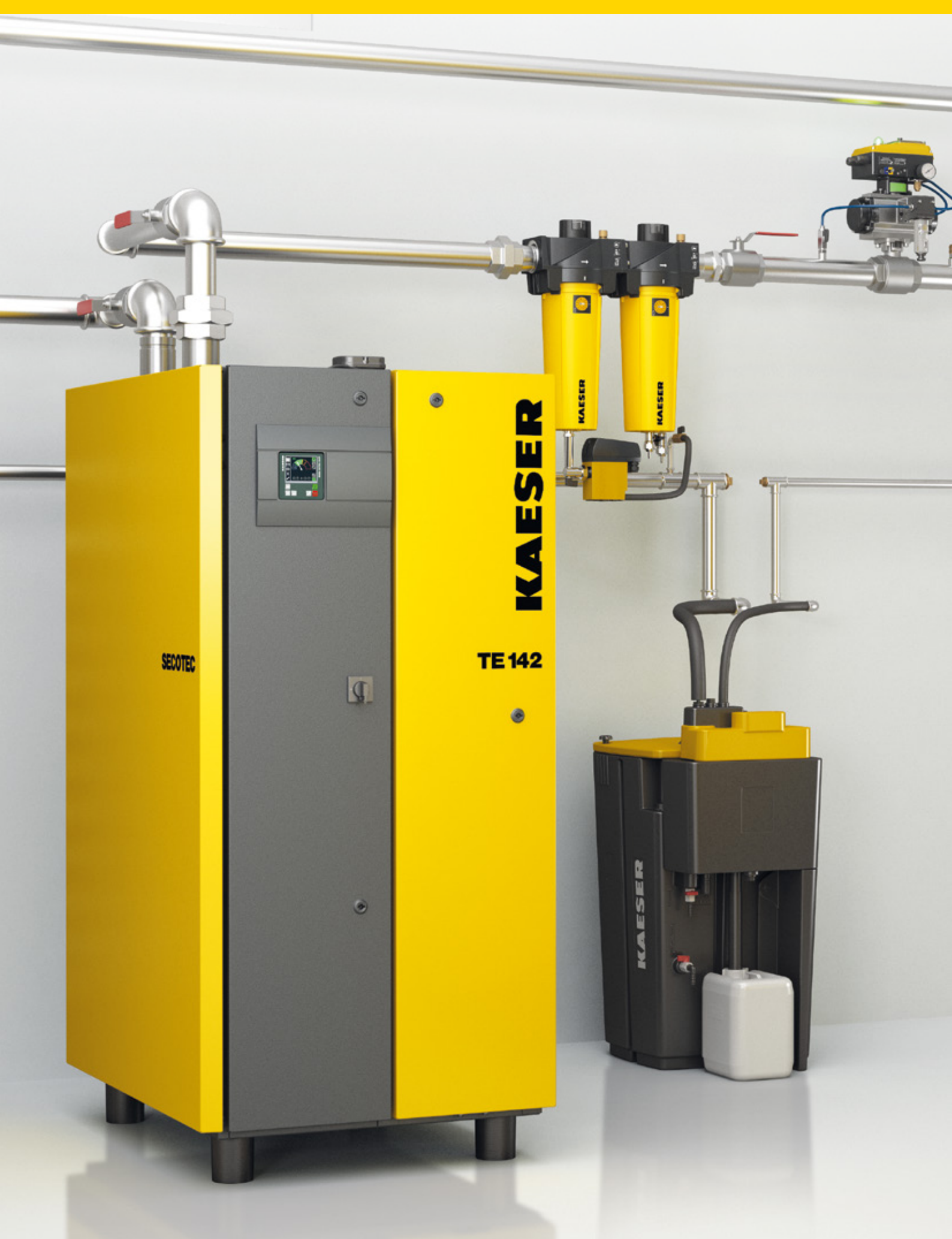
Fig. 2: Installation example for compressed air treatment with reirigeration dryer, coalescence filter and activated carbon filter plus air-main charging system
