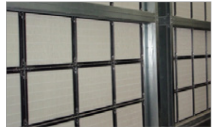
Fig. 2b: Cooling air filter system
