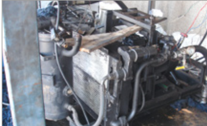
Fig. 1: Neglected compressed air station
