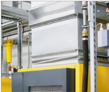
Fig. 2: Compressor ventilation connection with canvas duct joint
