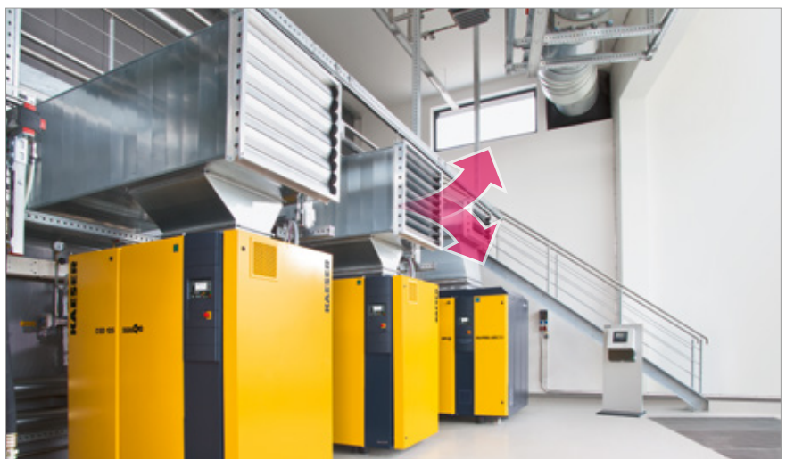
Fig. 3: Compressed air station with thermostatically controlled airflow
