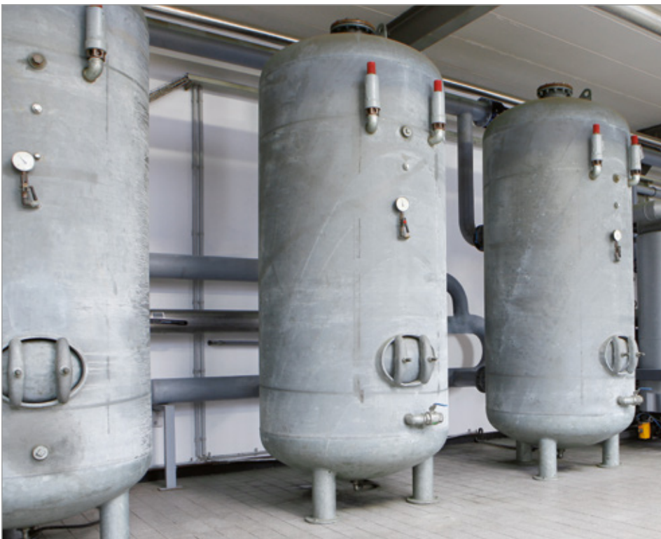
Fig. 4: Air receiver as buffer storage
